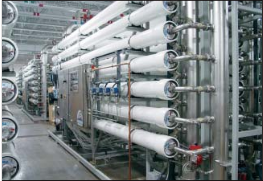
Minneapolis Water Works now operates an ultrafiltration system consisting of four trains with a total of 40 UF units, 36 of which are currently in service.
