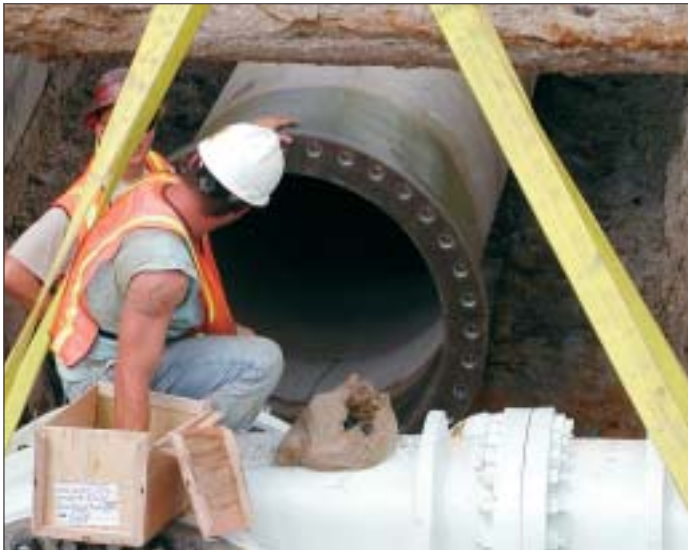
Fiberglass flanged connections made it easy to connect the pipes to the valves.
