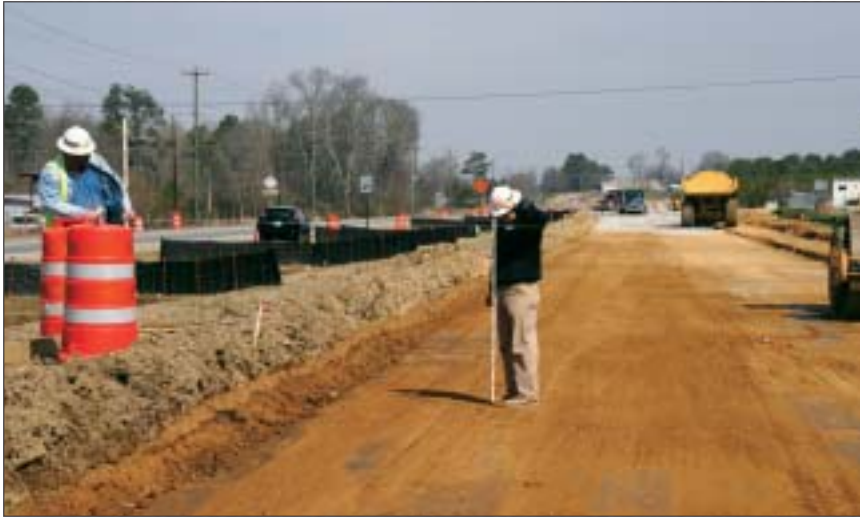
Without GPS, machine operators must rely on their experience and skill at reading stakes to carry a smooth, continuous grade.
