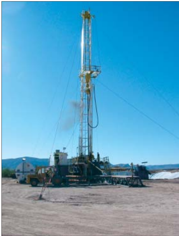
Eleven monitoring wells were drilled to monitor any changes in both water levels and water quality as the Hueco Bolson aquifer yielded its brackish groundwater.
