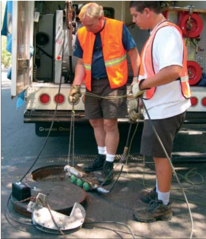
Ed Peterson, supervisor, and Ty Banagas, crew member, preparing to lower the main line camera into the manhole to conduct an inspection.
