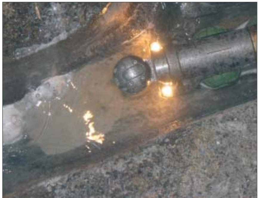
Camera on tractor in a main line at the manhole entry point. White foam is root remover that was administered after the camera spotted root problems in the line.
