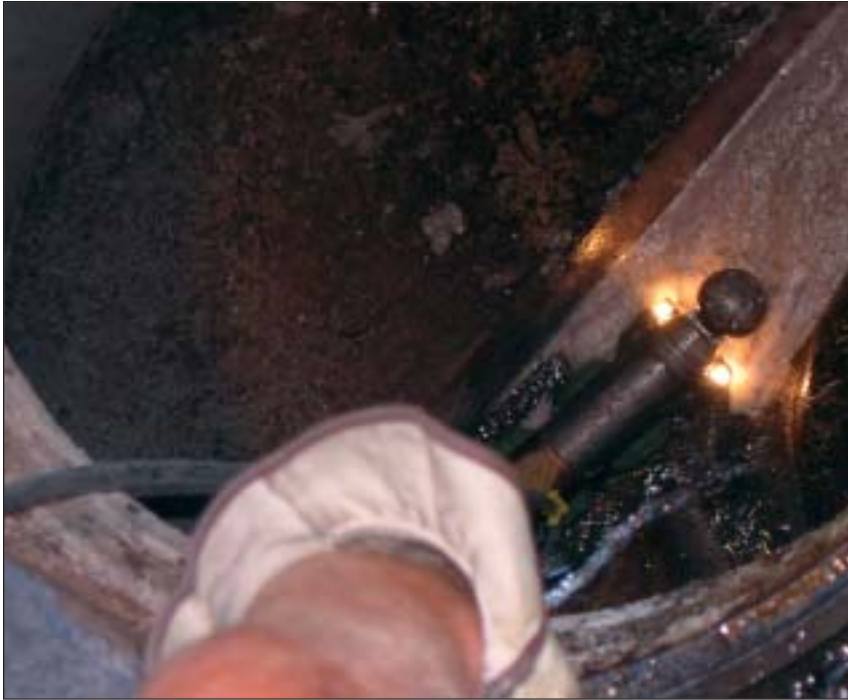
Crew member adding water to the main line after root elimination treatment has been administered to accelerate the root removal.
