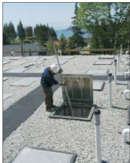
Woodard & Curran engineer Tom Hazlett checks a trickling filter at Vinalhaven's new 72,000-gpd wastewater treatment facility.
