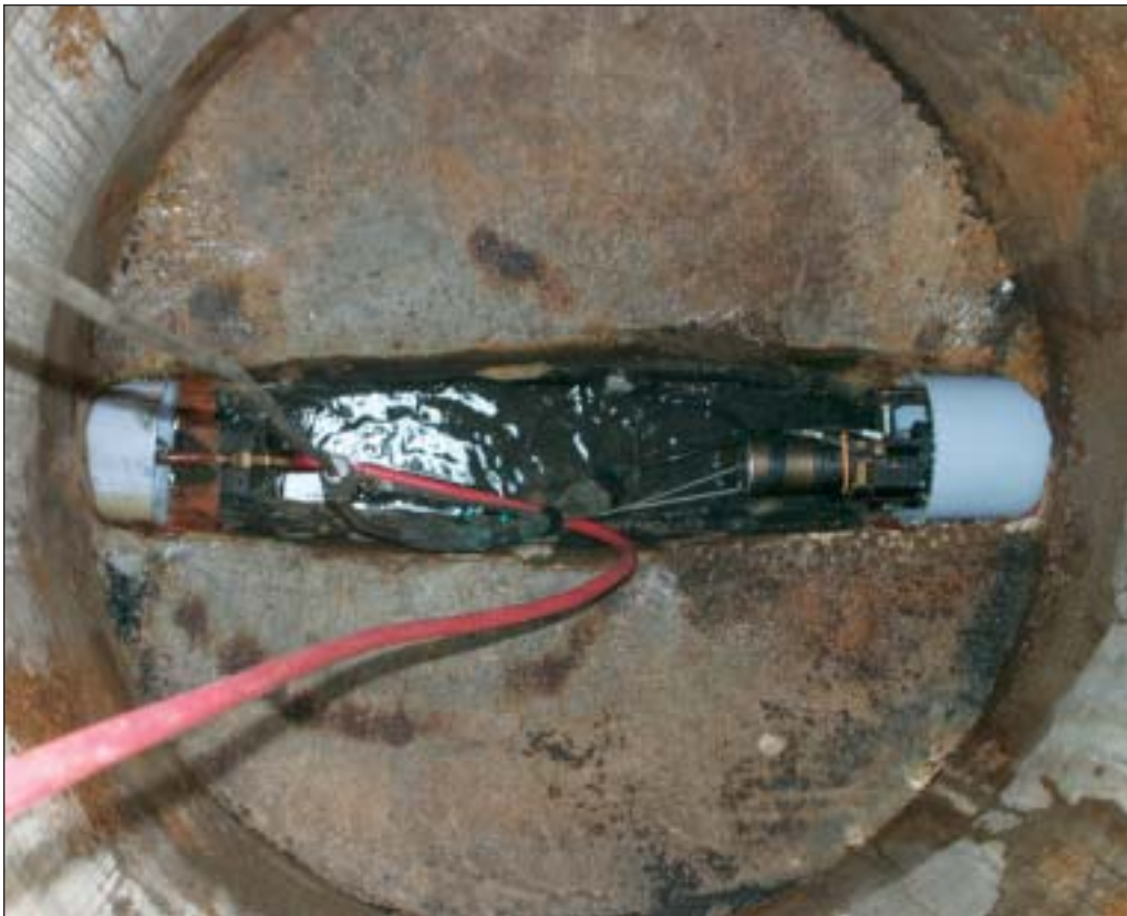
A look down a manhole reveals two steps in the Ultraliner repair process. On the left is the downstream end of a sewer line. It is plugged so that the steam and air can be pumped inside to inflate the PVC Alloy pipe to its full size. On the right, a remote controlled cutter is inserted into a repaired line to reopen the lateral connections. The entire repair process usually takes less than five hours.
