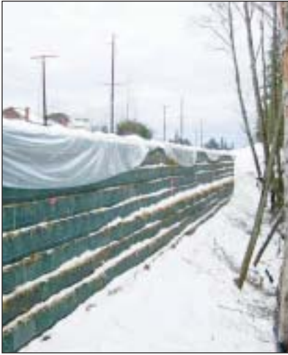
The finished wall in King County, WA, is shown here. In addition to MSE and embankment support, Geopiers can be used for shallow foundation support, slope stabilization, floor slab support, tank support, liquefaction mitigation, and uplift control.
