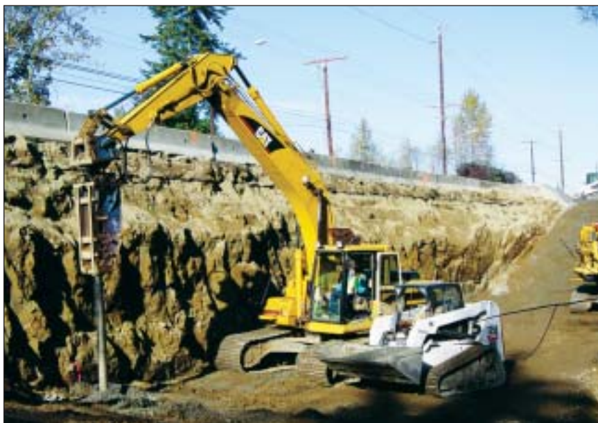
To stiffen the loose soils and increase the shear resistance beneath the wall, 88 production piers were installed 12 to 15 ft below grade in just four days.
