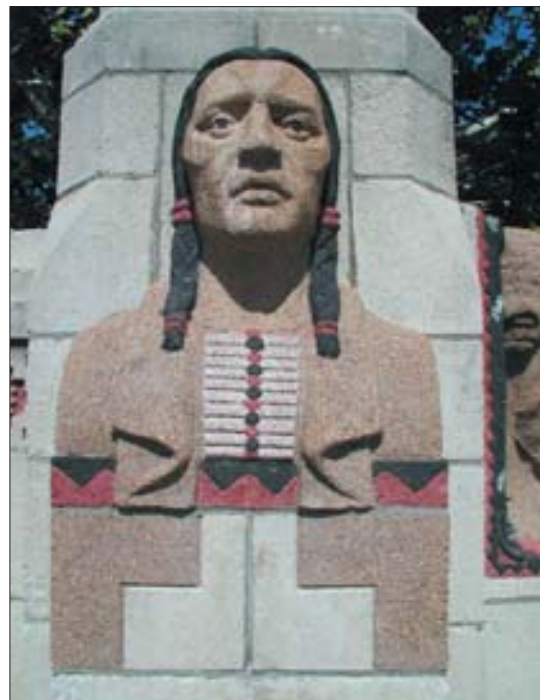
Sculptural elements on the parapets were restored. Often, pieces that were missing had to be replicated by artists using custom molds, carefully attached, and then shaved to fit.
