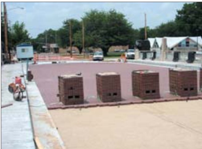
To maintain the historic aesthetics of the structure, the paving brick riding surface was replaced with similar-looking new bricks.
