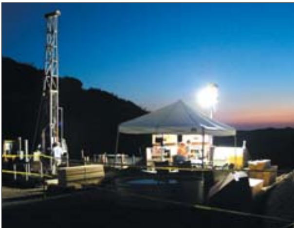
Tight scheduling on the project required one crew to drill at night.
