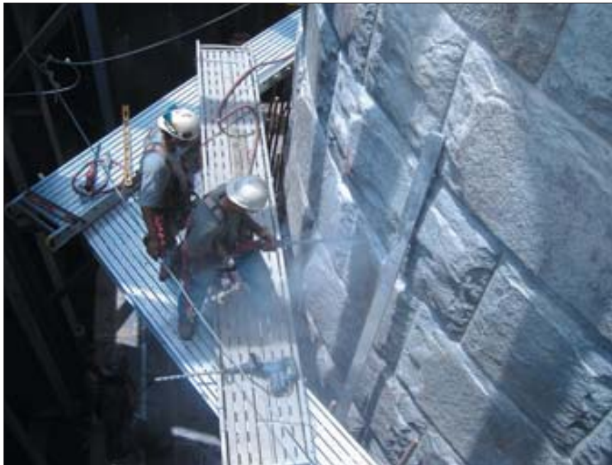
On the Huey P. Long bridge project, work areas and space were access-limited, making every place a hole had to be drilled a huge challenge.
