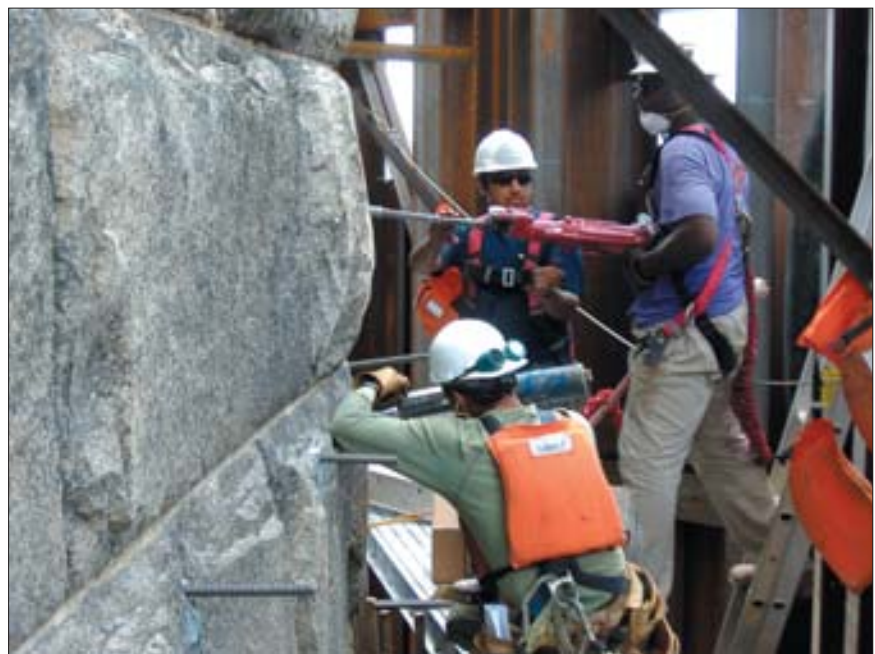
To tie the new concrete into the existing concrete, Chicago Pneumatic tools were used to install epoxy-anchored reinforcing steel into the existing piers.
