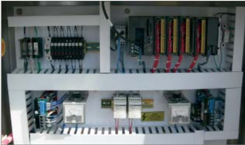
This is a sedimentation control panel. The smaller compact Modicon 948 PLC allowed the filter supplier to save cost while still being able to connect to the plant network.
