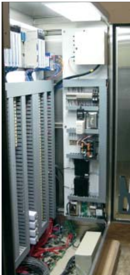
This is a typical Modicon Quantum programmable logic controller (PLC)-based main control system panel. Each control panel has a SCADA terminal inside for local viewing of all data points.
