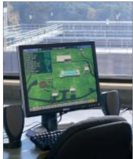
This is a view of a SCADA system in the control room overlooking the sedimentation basins. The SCADA system allows operators a full view into the process. SCADA stations are located throughout the facility for easy access.
