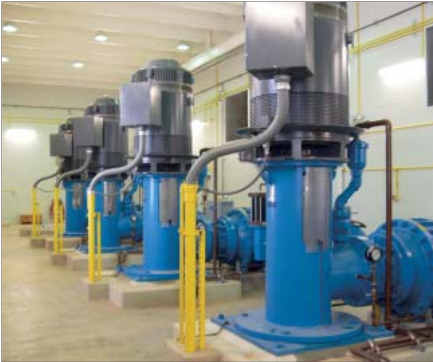
These are distribution water pumps controlled by Square D Model 6 motor control centers.
