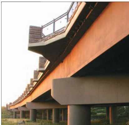
Pedestrians and bicyclists are able to enjoy the scenic landscape from overlooks included on several bridges.
