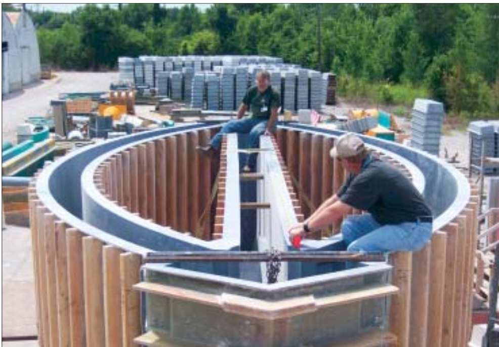
Unique archways and columns were created using intricate fiberglass reinforced plastic formwork.
