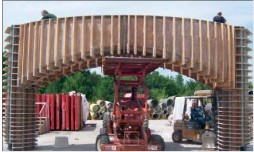
Fork-and-scissor lifts were used to safely lower down the large and bulky formwork.
