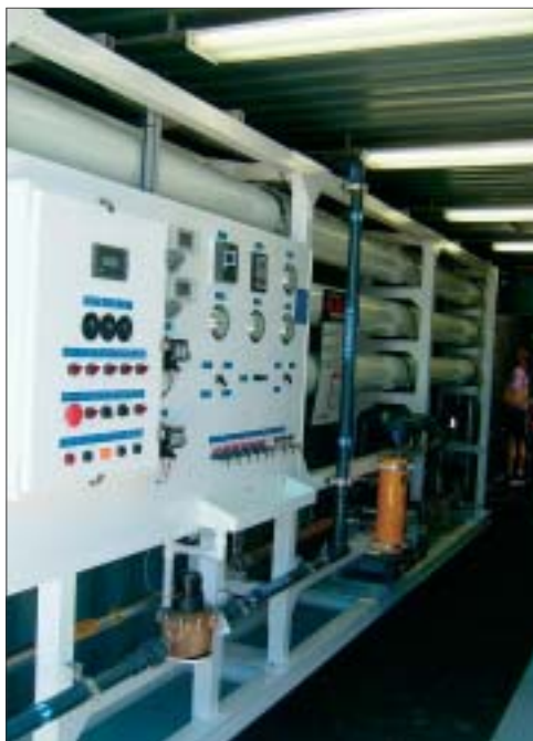
ADC seawater desalination facility in Pt Hueneme, CA.
