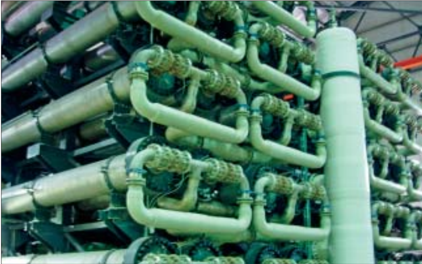
The pressure exchanger system of the Ashkelon seawater desalination plant, which currently is the largest system of this type in the world. This plant has broken the energy use barrier of 13.2 kWh/m 3 established by previous projects for intake salinity in the range of 38 to 41 ppt.
