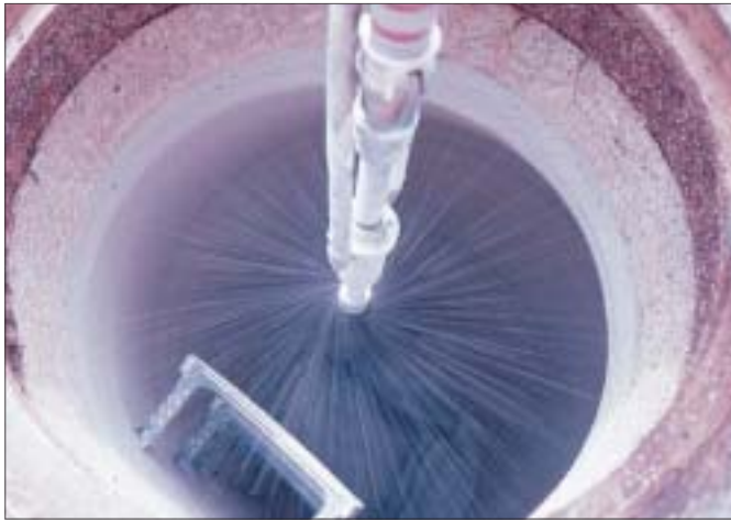
The majority of lining applications within Lowries Run manholes utilized spincasting technology from ground level.
