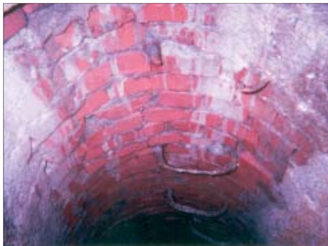
The necessity for rehabilitation is evident in this Lowries Run manhole.
