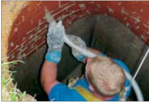
A cement-based resurfacing material is pumped into open mortar joints within manhole chimneys.
