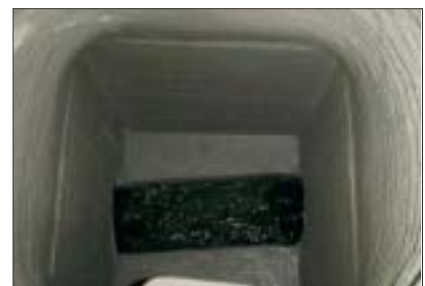
Typical Lowries Run manhole, post-application: Sauereisen's lining completely restores and seals the concrete vaults and brick chimneys.
