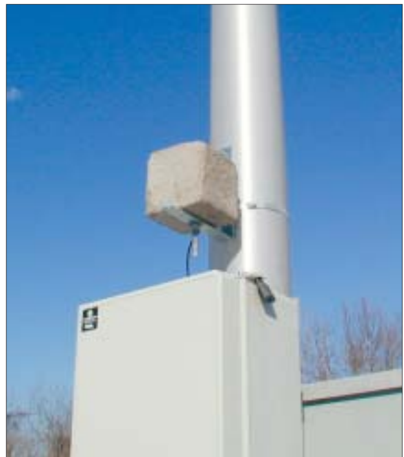
A typical RWIS station tower located in the median of I275 near Cincinnati (top). Bottom, close-up of a bridge deck simulator.
