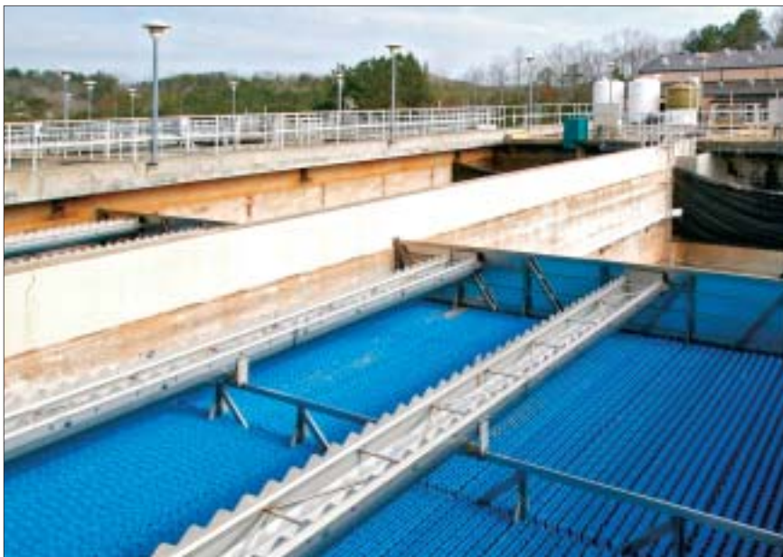
The renovation of the facility's existing sedimentation basins includes adding inclined tube settlers.
