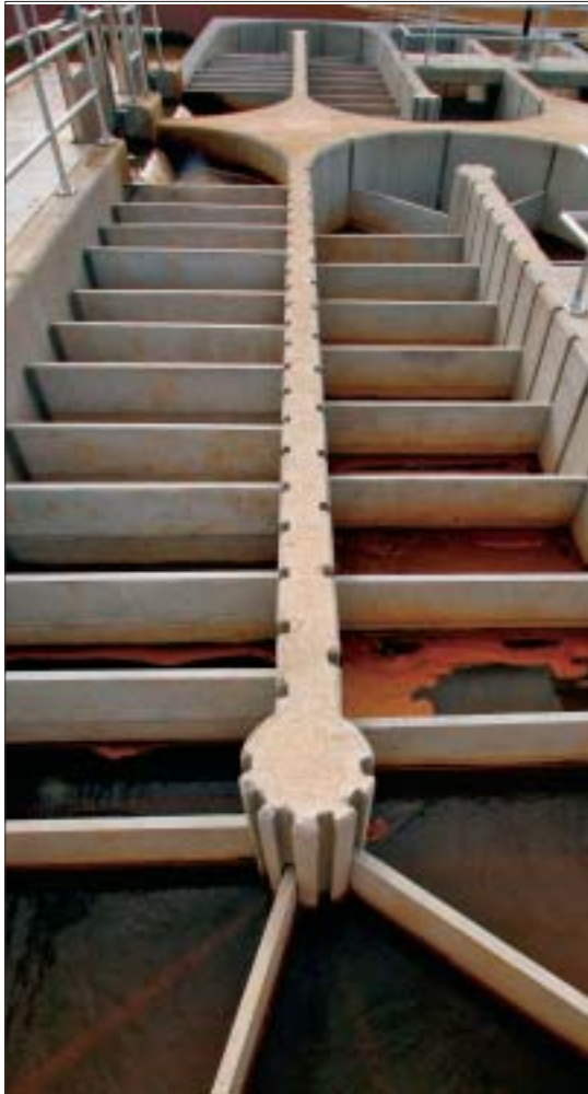
The drinking water facility's eight new flocculation basins include flocculator baffles, a diffuser wall, a floating baffle, and a head baffle.
