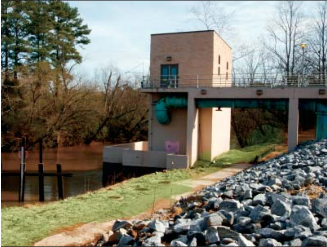
To augment the plant's pumping capacity, two pumps were added to Raw Water Pump Station No. 2.
