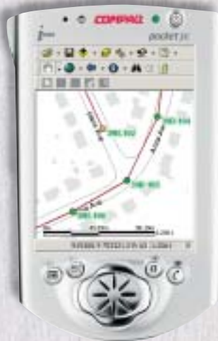
Field workers used handheld computers with a GIS to collect information during manhole inspections.
