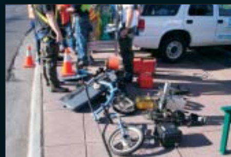
PPIC personnel prepare to enter Conduit No. 30 and assemble PipeRider—a self-propelled RFEC/TC inspection tool.
