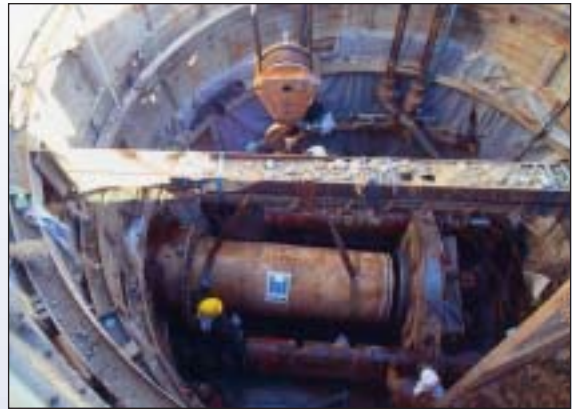
Push-together assembly with leak-free joints helped shorten the Lafayette, CO, project duration. High strength pipes allowed direct jacking in a few critical areas.
