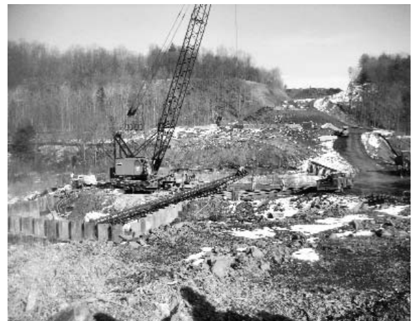
A temporary causeway was built to mitigate the impact of bridge construction.
