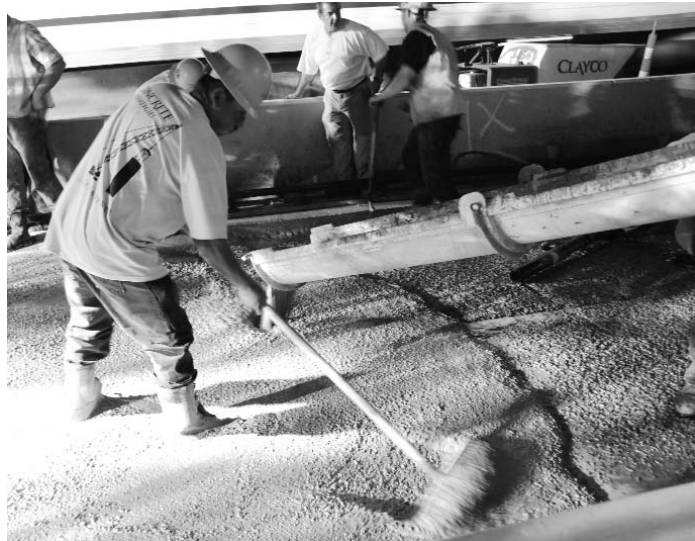
An eight- to nine-in. slump was allowed at discharge, a seemingly high slump that produced a cohesive concrete that was easy to place.
