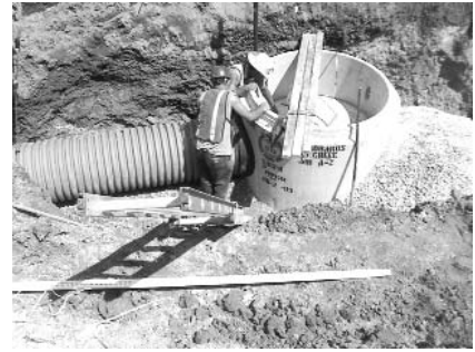
SaniTite HP pipe is being used in a $1-million sewer project to prepare vacant land in the Kentucky heartland for future development.
