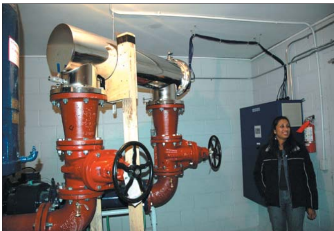
During the study, Staab Construction, a Marshfield, WI-based contractor, temporarily installed the UV systems on wood cribbing at the wellheads like that shown here.
