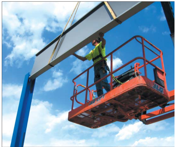
Light weight of the composite sound barriers translated into savings because of smaller crew sizes and reduced truck shipments to the work site.
