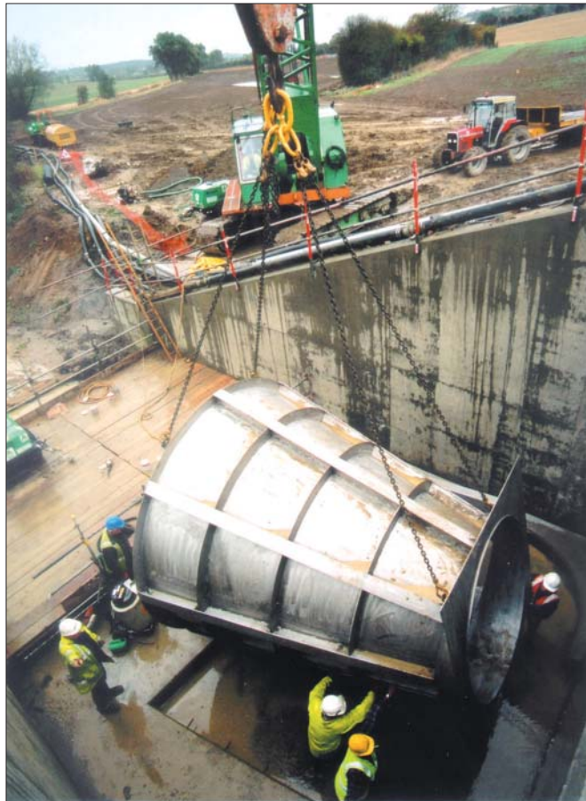
Installation of a large vortex valve, whose design—a snail or conical shape—cause high flows to initiate a vortex within the valve, restricting the flow of water out of the device.
