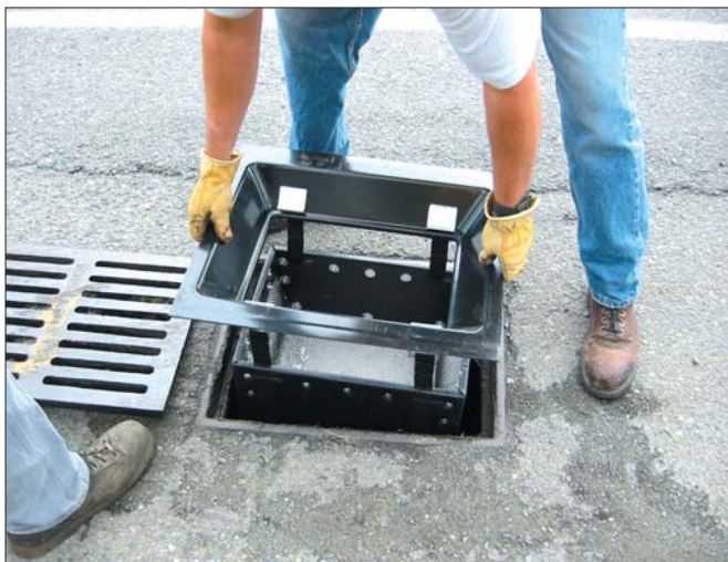
Long Beach and Norwalk fitted critical storm drains, such as this one, with high-technology filtration systems filled with Smart Sponge Plus, which contained the antimicrobial capability to protect recreational beaches.
