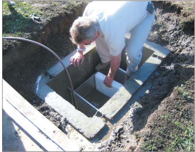
Westchester County (NY) Airport has installed catch basin filters in critical storm drains to protect waterways surrounding the airport from polluted runoff.
