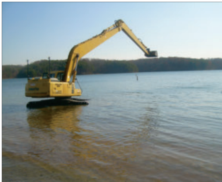
Outfitted with spill kits to protect against oil leaks, the excavator waded out until water reached the top of the tracks, but not the cab.
