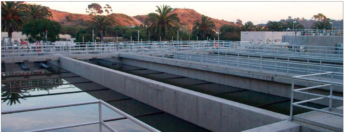
The San Elijo Water Treatment Plant produces 2.5 mgd of recycled water. Secondary clarification process tanks are about 220,000 gal. each. Average treatment time in the tank is slightly over five hours.
