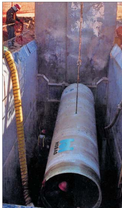
A 20-ft length of 60-in. diameter HOBAS pipe is lowered into the jacking pit during the Oklahoma City sewer construction.
