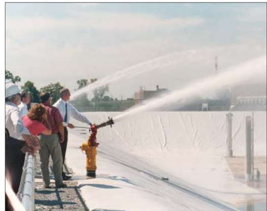
Indianapolis Mayor Bart Peterson visits the completed equalization basins at the Belmont advanced wastewater treatment plant.
