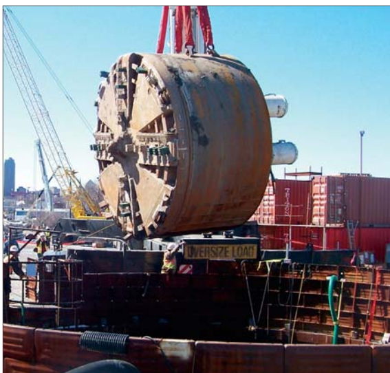
Equipment used to bore a nine-mile long tunnel that will transport CSOs to city treatment plants is lowered into place.
