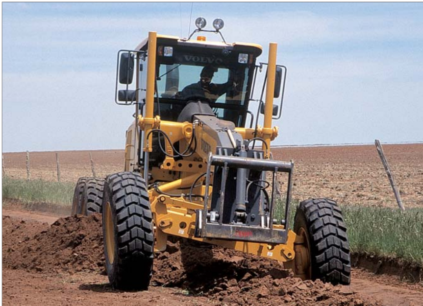
Graders make multiple passes to move dirt from both ditches up onto the road, losing the roll as it reaches the center.
