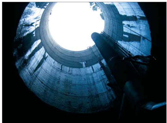
At the Custer Avenue CSO, a new dechlorination facility will treat chlorinated flows coming from the Boulevard regulator.
