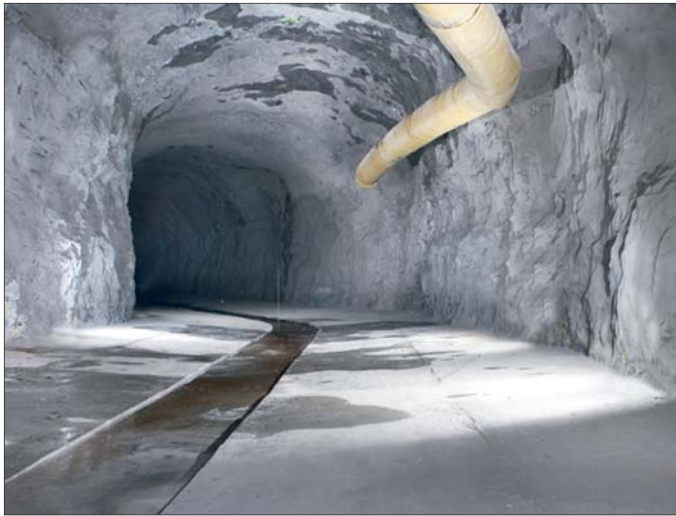
Combined sewer overflow (CSO) storage and transport tunnel.
