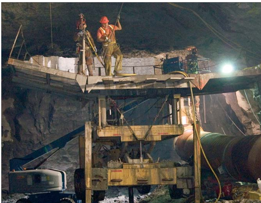
Ten-mgd cavern is a linear storage facility excavated out of granite and connected to the existing tunnel and shaft.
