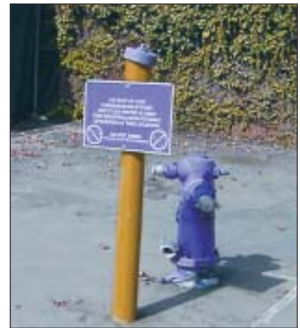
Recycled water hydrant is painted purple and outfitted with different connectors than on a standard hydrant.
