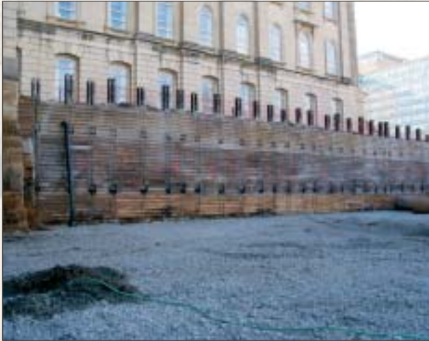
Completed soldier pile and lagging wall (with tiebacks) for northwest vault construction, looking south.
