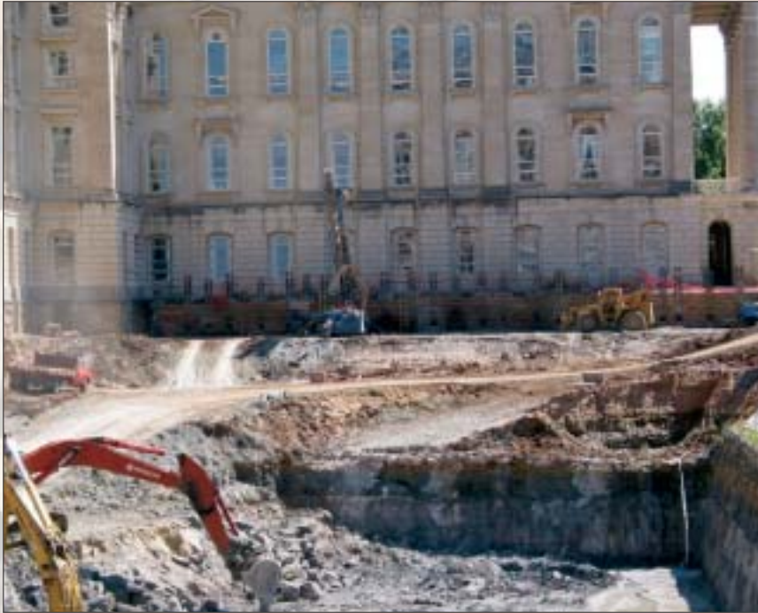
Geotechnical specialty contractor installing tiebacks for soldier pile and lagging wall, northwest vault.
