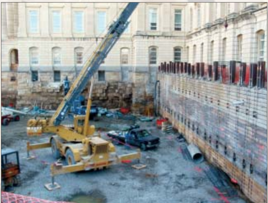
Completed soldier pile and lagging wall — with tiebacks— for northwest vault construction, looking east.
