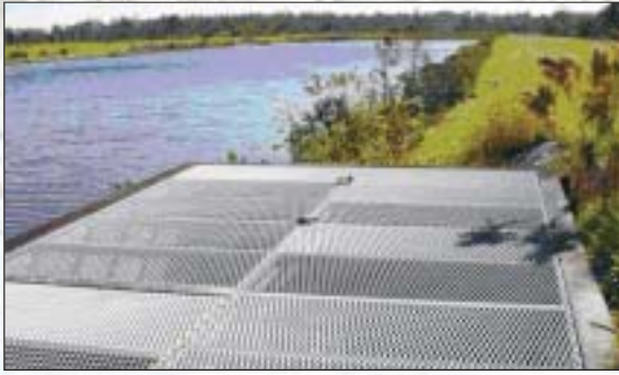
Control structures must be barricaded to be sure the carp remain in the treatment area.
