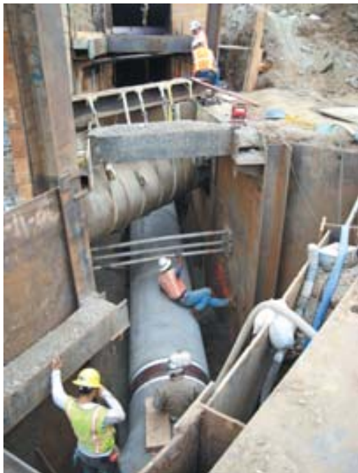
Wet and dry utility excavation and relocation—while keeping services running—was a construction management challenge requiring months of 24/7 planning, permitting, sequencing, monitoring, and communication. Photo credit: PBS&J
