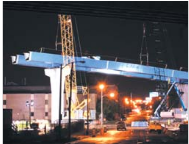
Supported by predominantly high performance steel, the interchange’s ramps and bridges are considered one of the nation’s safest highway structures.
