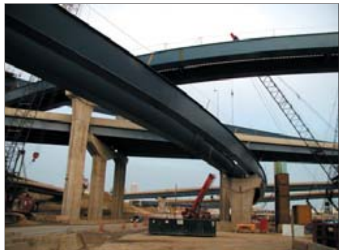
All curved multi-span twin steel composite box-girder bridges up to 2,400 ft long, the eight high-level system ramps were the centerpiece of the project.
