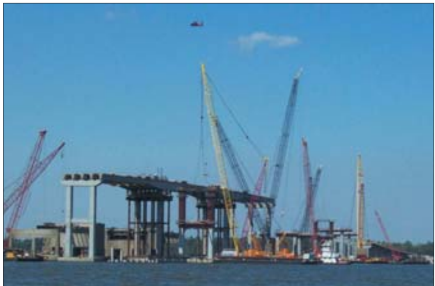
The westbound main navigation span on the US 90 Bridge over Biloxi Bay was set on April 24, 2007.
