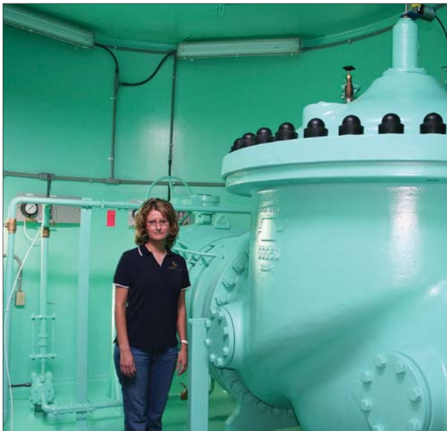
The 36-in. pressure reducing valve in assembly with an EFI employee indicates the size of this project.
