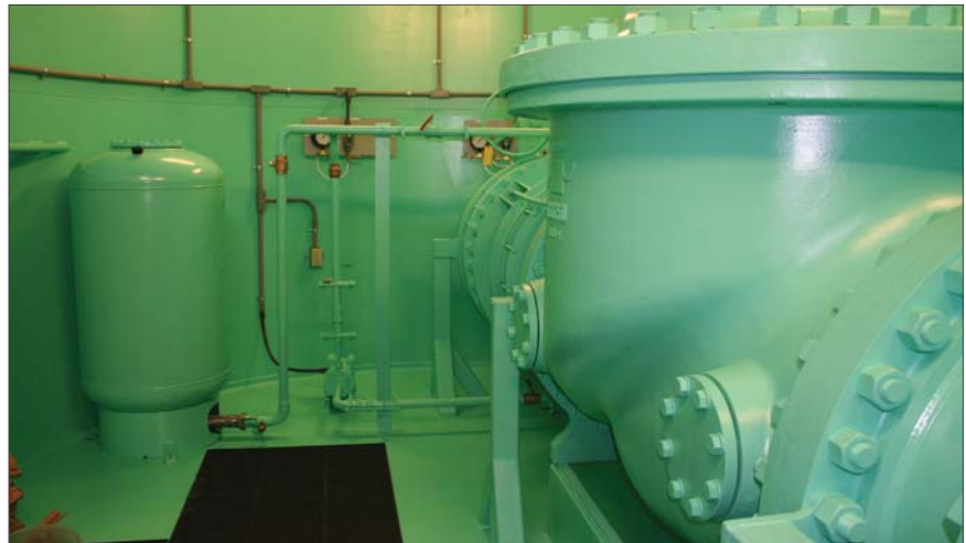
Shown here are the pilot water system tank, pump, and piping. Behind the 36-in. control valve is the breakaway coupling included to facilitate valve withdrawal if ever required.
