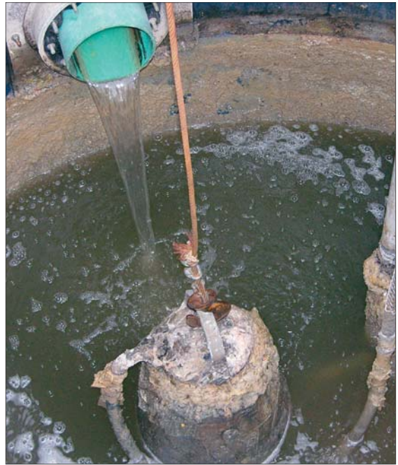
Hospital discharge from the blue pipe is transferred to the wastewater treatment plant by two pumps.
