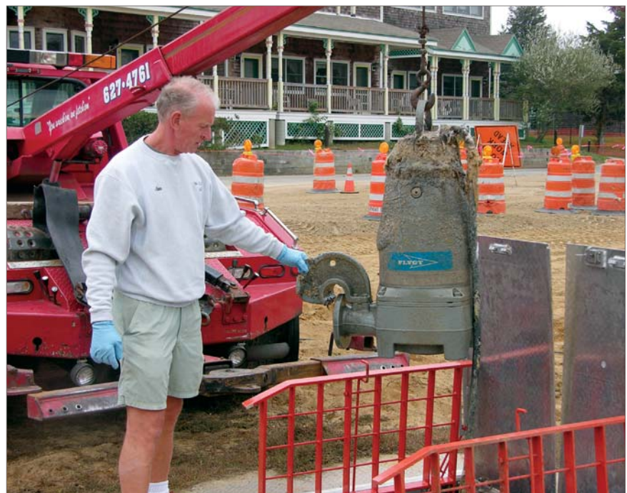
First time pump is removed from pit for visual inspection; it is clean and unclogged. The old hospital is visible in the background.
