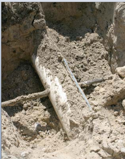
Workmen accidentally hit a Fripp Island vacuum sewer collection line dead center when installing cable.
