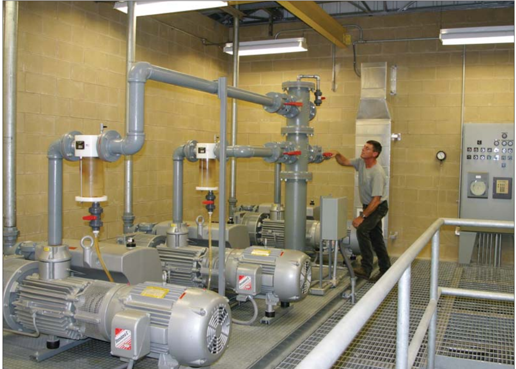
Vacuum sewer stations provide a clean, odor-free working environment, and because vacuum sewers are a closed system, workmen never come in contact with raw sewage.
