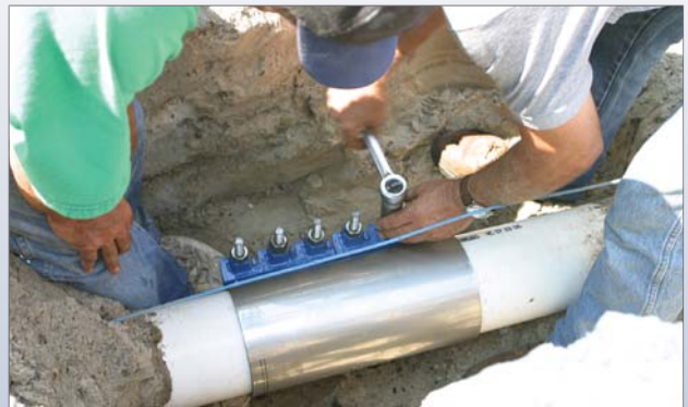
Repairing the damage was relatively simple, as the shallow depth of the line made access easy. A full-circle clamp was applied and the line was back in service in less than an hour.
