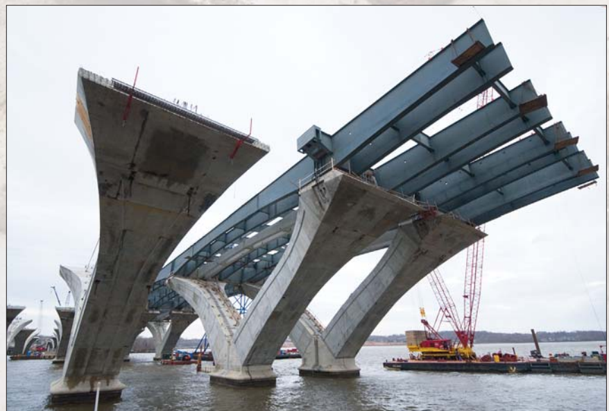
Clearance under the new span is 20 feet higher than the old bridge, significantly reducing drawbridge openings. Photo by David Sailors.
