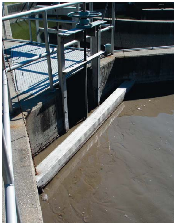
To improve internal hydraulics and increase mixing in the ditch, in 2005 a baffle was installed in the oxidation ditch.
