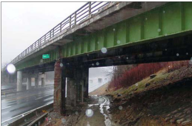
New York State Department of Transportation inspectors discovered that the outer columns and pedestals of two of the piers had deteriorated badly.
