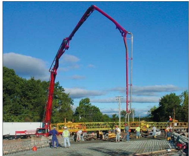
All phases of construction were affected by the dramatic skew of the bridge — 58.5 degrees.
