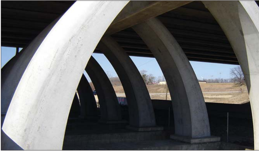
University Avenue Arched Pier Bridge over I-74, Peoria, IL. Photo courtesy of Alfred Benesch & Company
