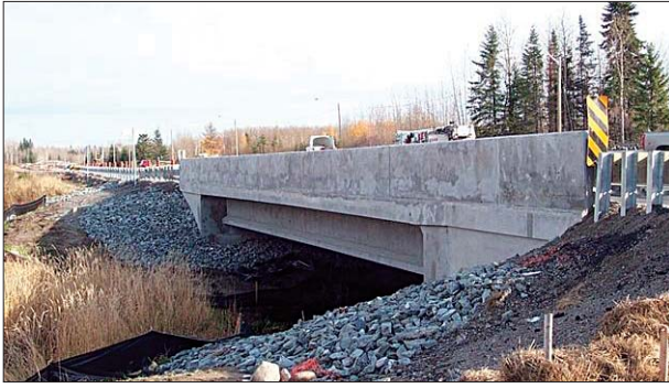
Moose Creek Bridge, Timmins, Ontario, Canada. Photo courtesy of Ministry of Transportation, Ontario/Stantec Ltd./Precon Inc.
