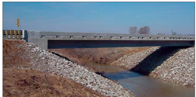
Wapello County Mars Hill Bridge, Wapello County, IA. Photo courtesy of Rich Sanders/GPA
