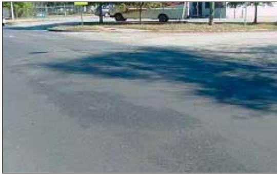
Delamination of Rio Grande Pavement
