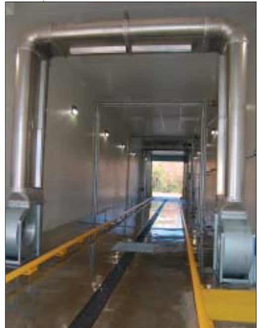
Empty wash system awaits...
