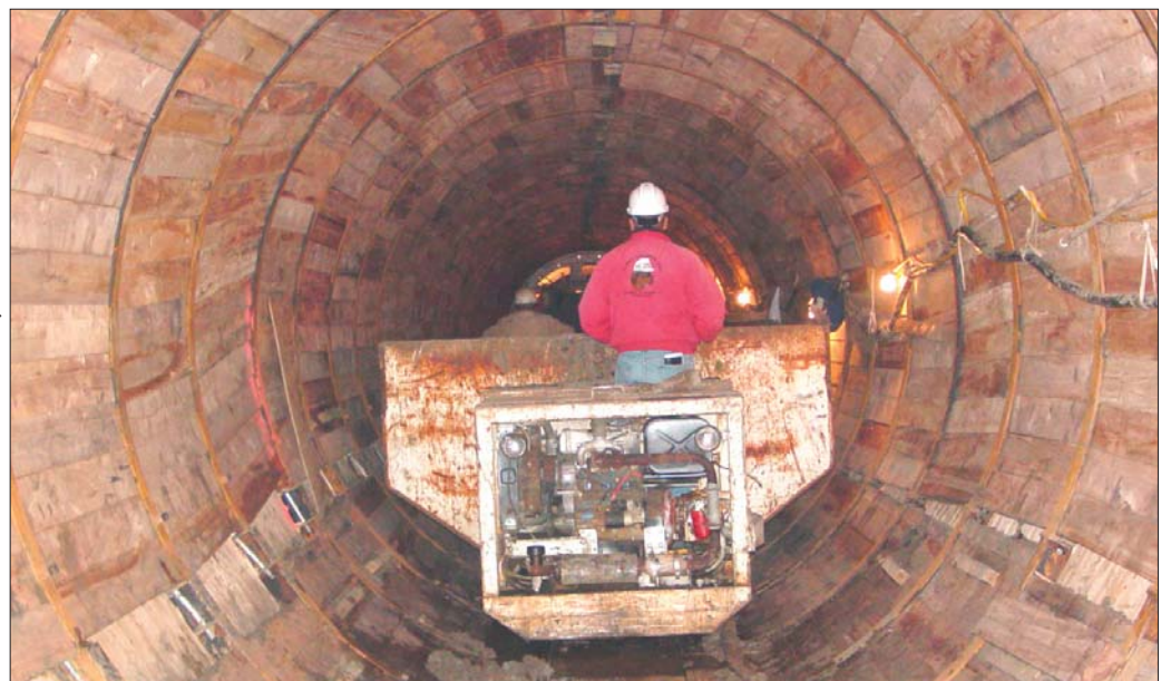
In two-pass tunnel installation, CCFRPM pipes are cost-effective since the high-strength, thin-walled product permits a smaller primary tunnel. Note the steel ring beams and wooden lagging used to construct the primary tunnel in the two-pass system.
