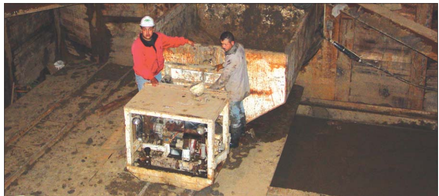
In Grand Prairie, a rail system was established to remove spoil from the tunnel and later install the new pipe.
